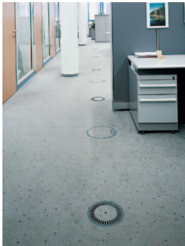
Figure 5: NTK floor twist outlet in an office building
