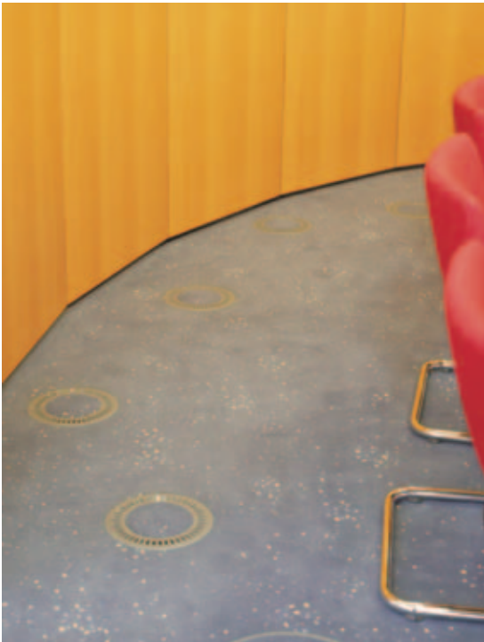
Fig. 3: Floor displacement outlet in a meeting room
